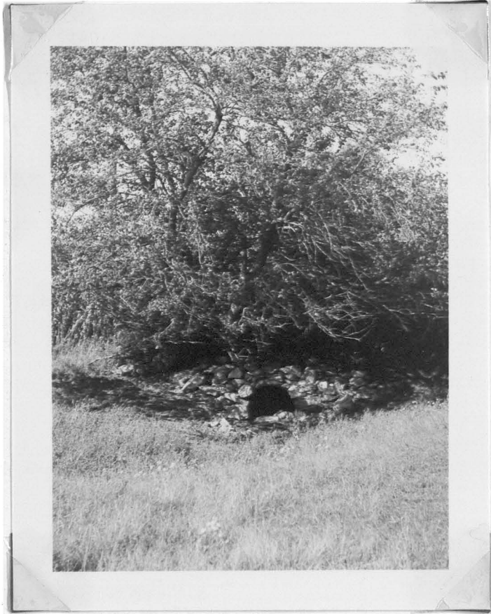
Fig. 17. A mulberry tree growing from the end of a rock reinforced railroad culvert. Many ripe mulberries fell on these rocks and were eaten by the spotted skunks living at this place.
